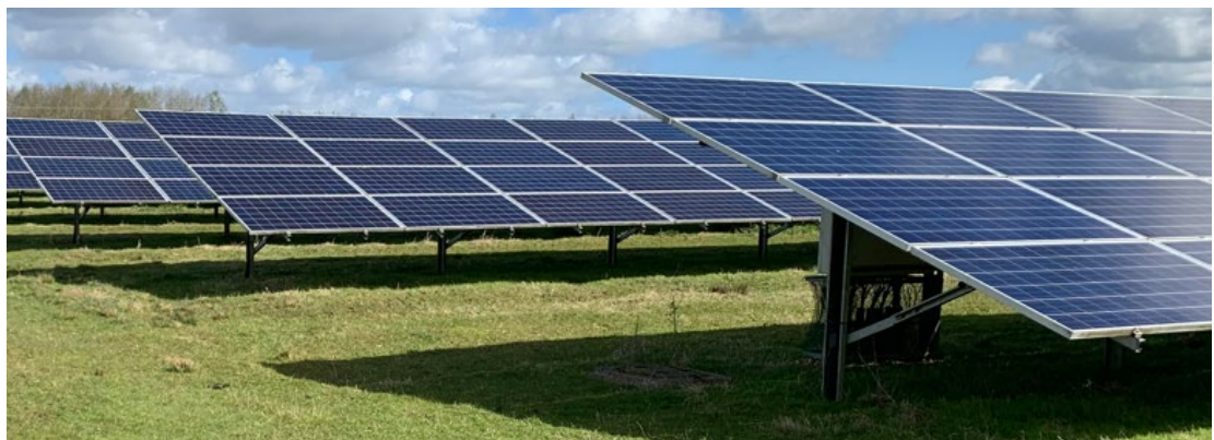
Photo 15.23: Panels Array Showing Gaps Between Panels
