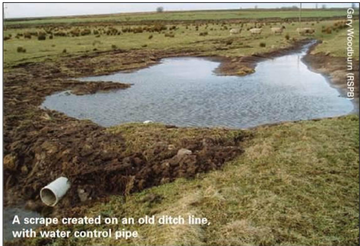
Figure 5: Scrape Connected to Ditch Line
