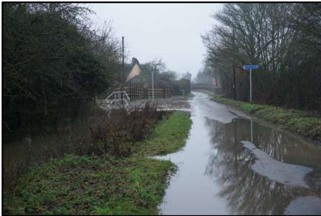
Church Lane, February 2026 flooded and the culvert to the left is full to the brim as is the field pond to the right.
