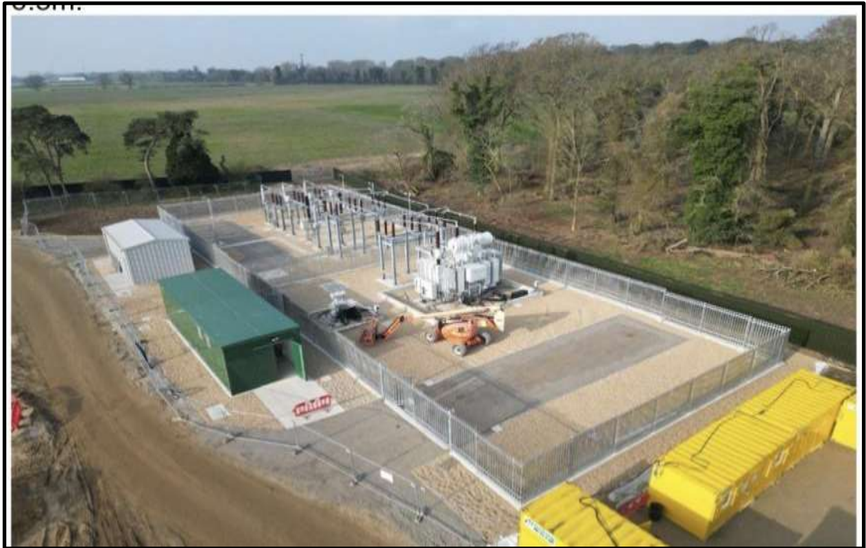
Image 132/33kV Substation (single transformer) East Pye Solar
