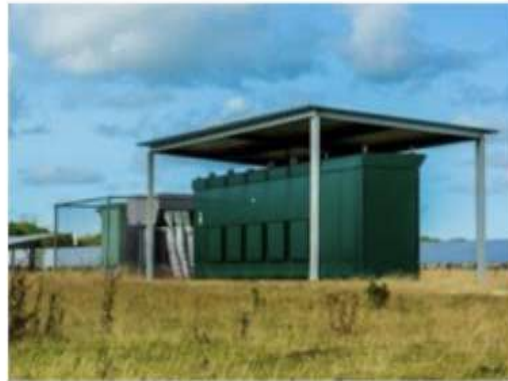
Image 4 Central Inverter Unit
