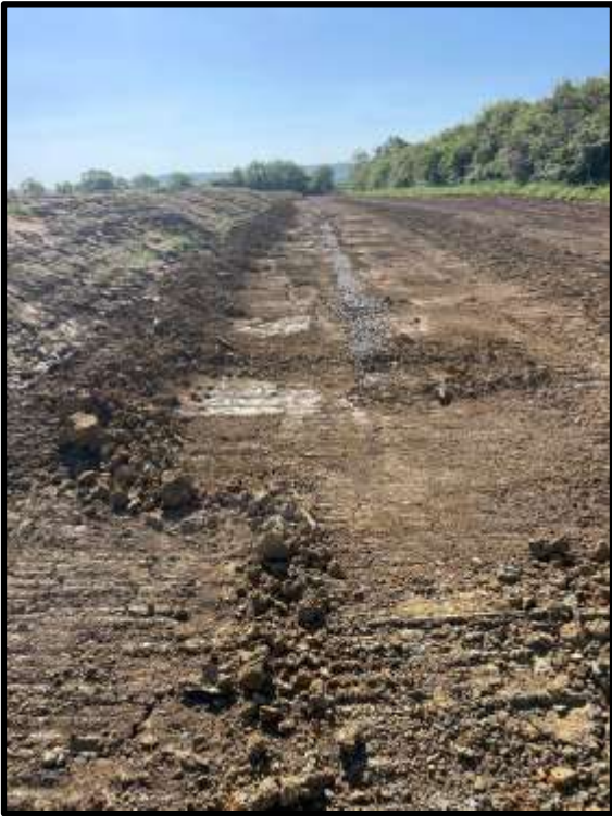
Melton -Destruction caused when trenching cables and drainage
