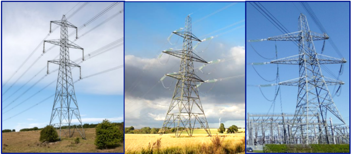
Plate 4.2 - Suspension Pylon (Left), Angle Pylon (middle), and Terminal Pylon (Right)
