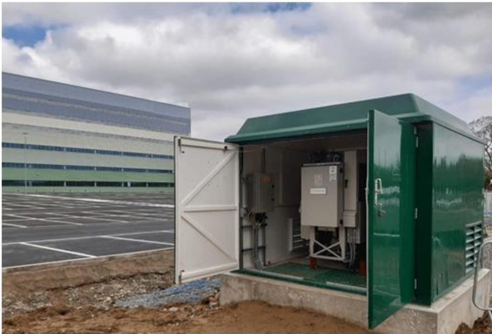
Plate 2-3: Example of Above Ground Infrastructure – Pumping Station Kiosk
